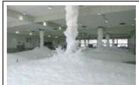
Foam Suppression System
